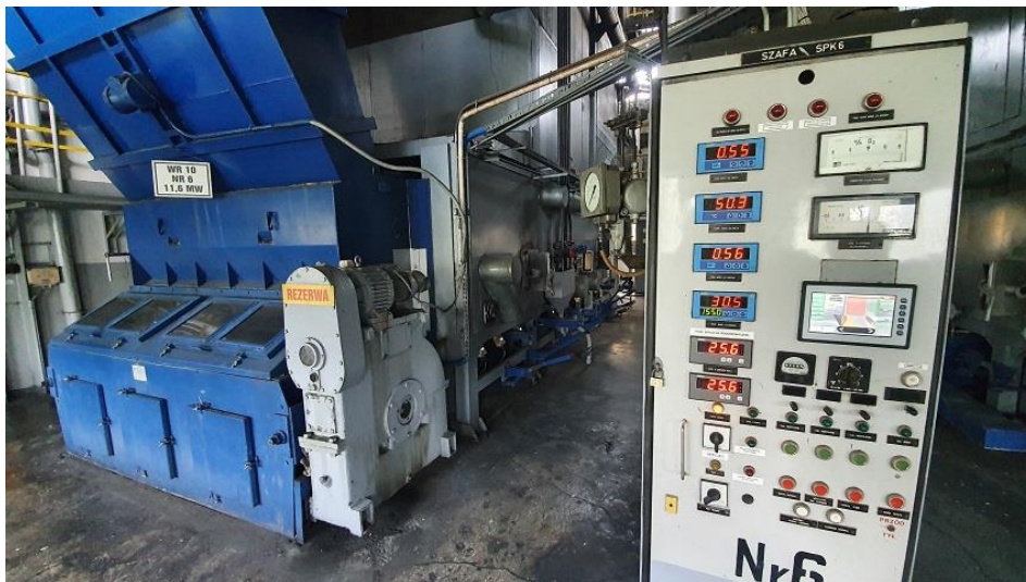
Figure 2-79. A 11.6 MW coal boiler facility 41
